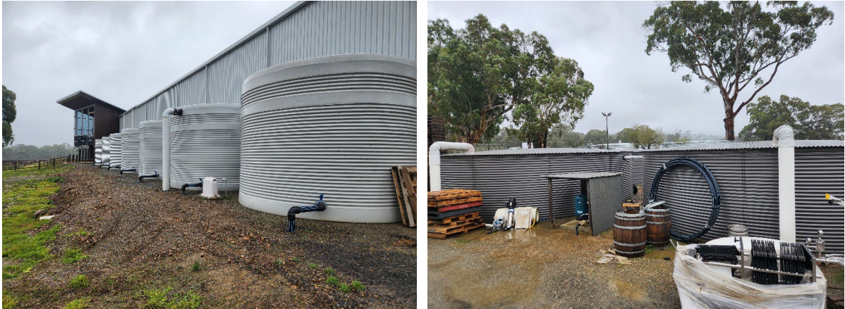
Figure 2 Rainwater storage tanks at Yangarra in McLaren Vale. Yangarra has 500kL of storage capacity.
